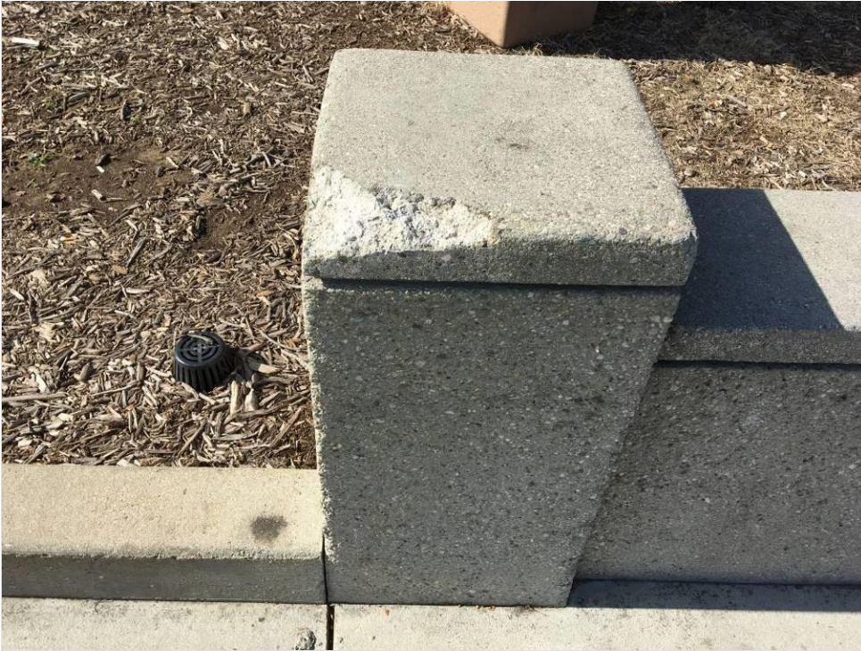
Photo 31 – Spall at concrete landscape wall probably caused by impact damage.
