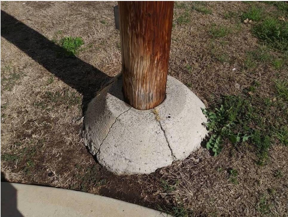
Photo 32 – Existing wood power pole at south end of building. Note cracks in concrete foundation.
