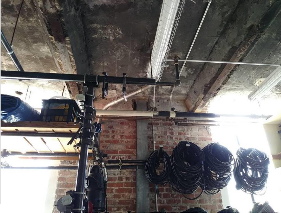
Photo 29 – Underside of concrete mezzanine slab located at the south end of the building. Note significant water staining and missing concrete at the bottom of the steel I-beams.
