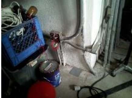
E-14: Open junction box in utility room
