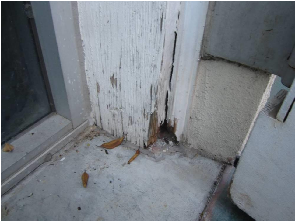
Photo 18 – Wood decay at the base of the wood door frames.
