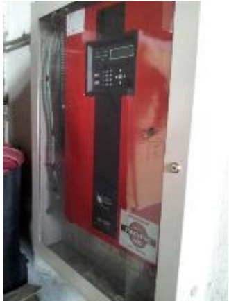
E-12: Fire Alarm Control Panel
