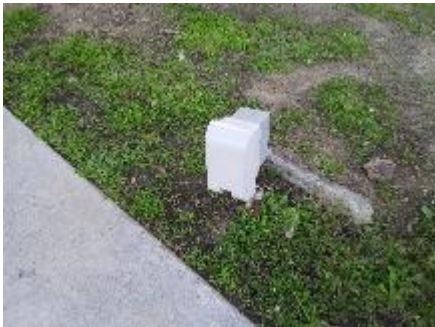
E-30: GFCI outlet near entrance not working
