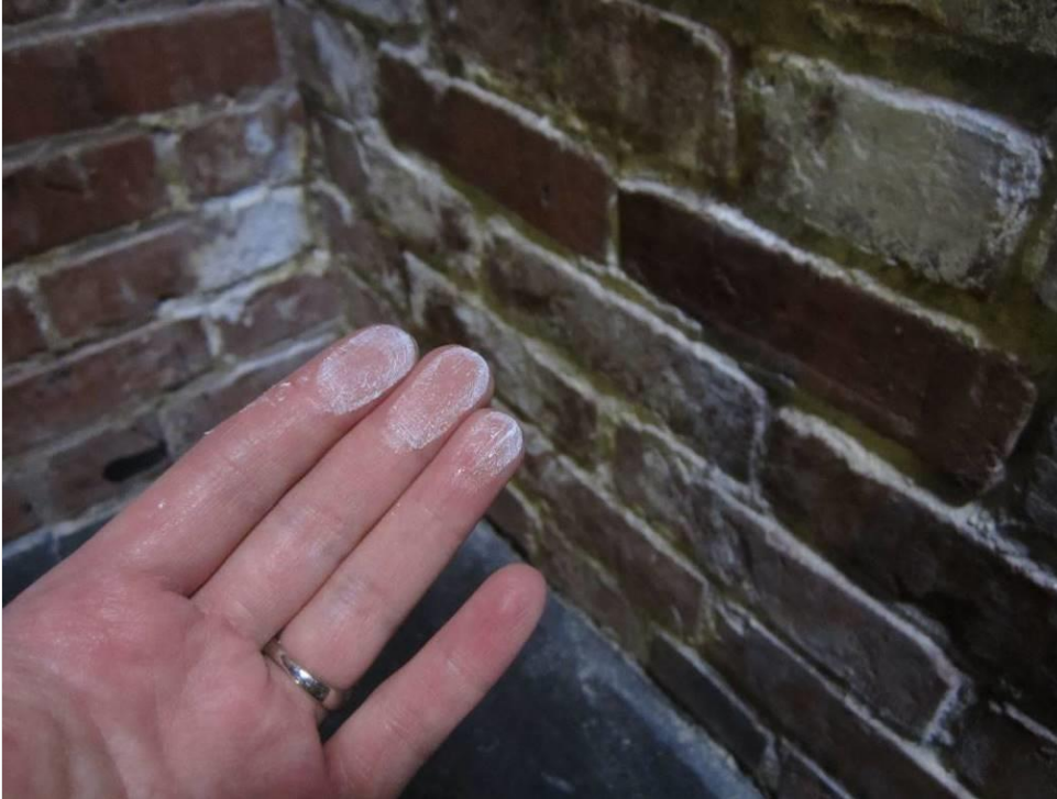
Photo 11 – Efflorescence at interior brick masonry wall.
