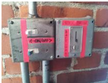
E-1: Light switches near front entrance
