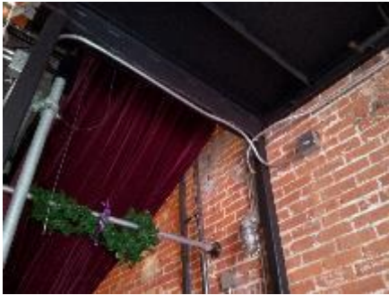
E-3: Vapor tight wall sconces found in both 1 st and 2 nd floors
