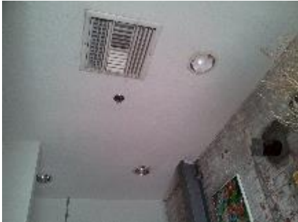
E-19: Downlights in 2 nd floor restroom
