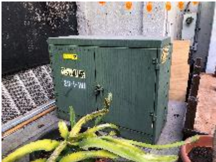
E-32: Utility Transformer
