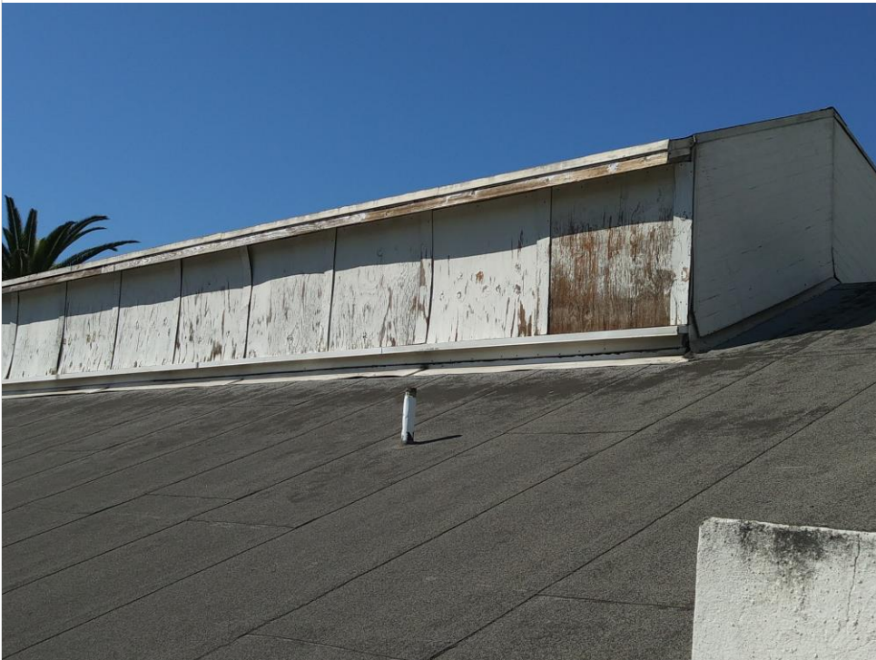
Photo 20 – Existing roofing membrane and view of raised monitor roof from the east.
