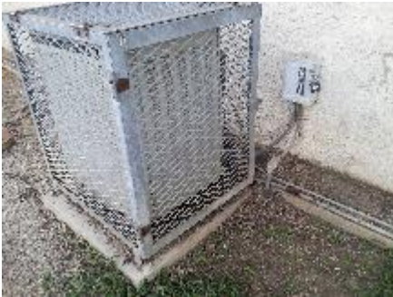
E-35: Exterior AC Unit with disconnect
