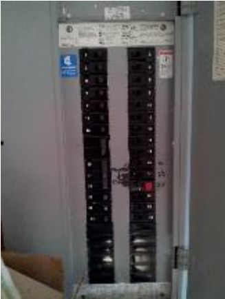
E-21: Panelboard "A" in office room
