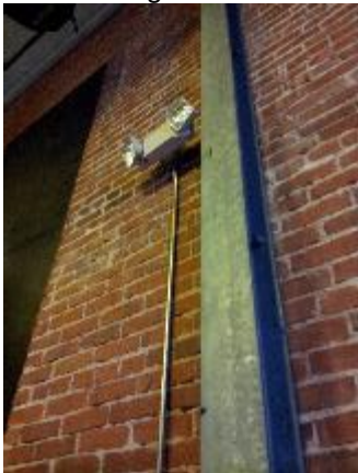
E – 29: Emergency lighting in performance hall
