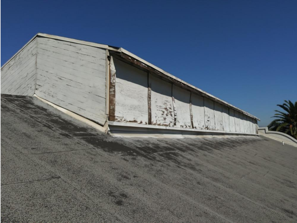
Photo 19 – Existing roofing membrane and view of raised monitor roof from the west.
