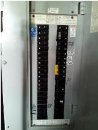
E-9: Panelboard "B" in utility room
