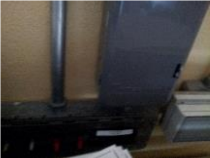
E-23: Switches in office room
