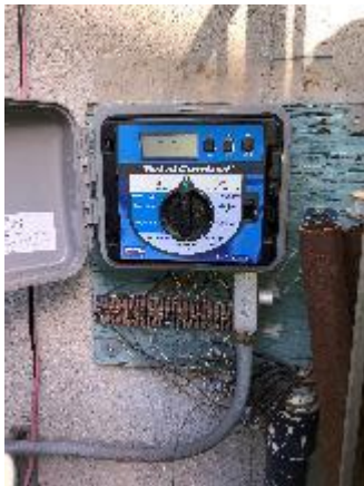
E-36: Exterior irrigation controller
