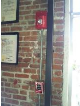
E-4: Fire alarm pull station and strobe
