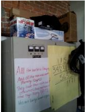
E-10: Inverter not in use
