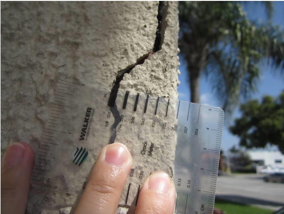
Photo 8 – Width of vertical crack measures 1/8 inch in width.
