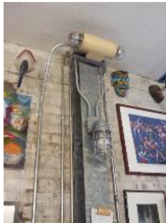
E-24: Emergency lights in open office area
