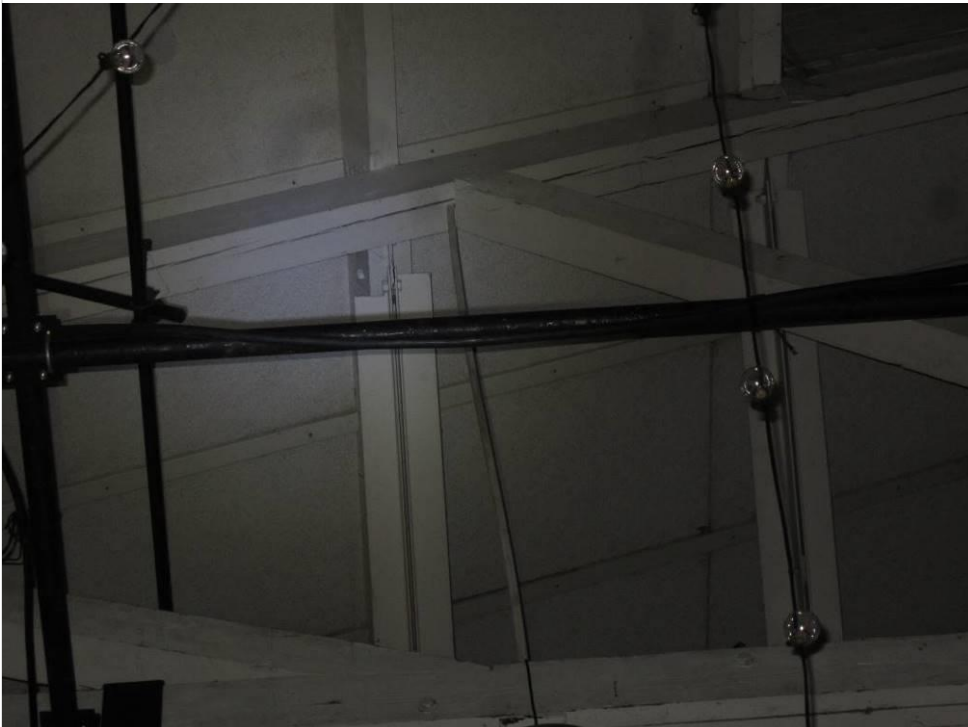
Photo 28 – Split is wood truss member.
