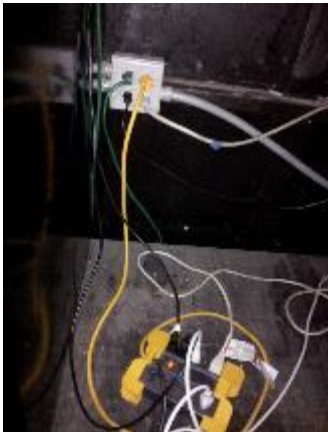
E-26: Quad outlet in control room
