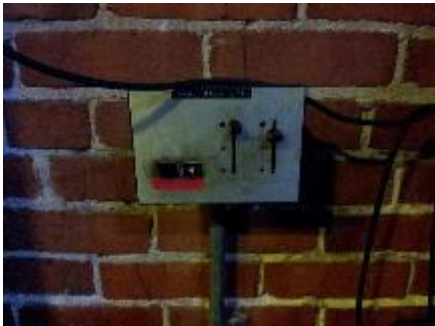
E-27: Dimmer switch controlling (5) 2x4 light fixtures
