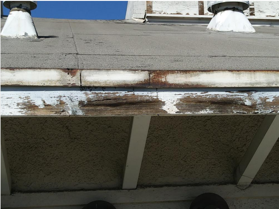
Photo 24 – Deteriorated wood fascia board and corroded edge flashing at roof eave.
