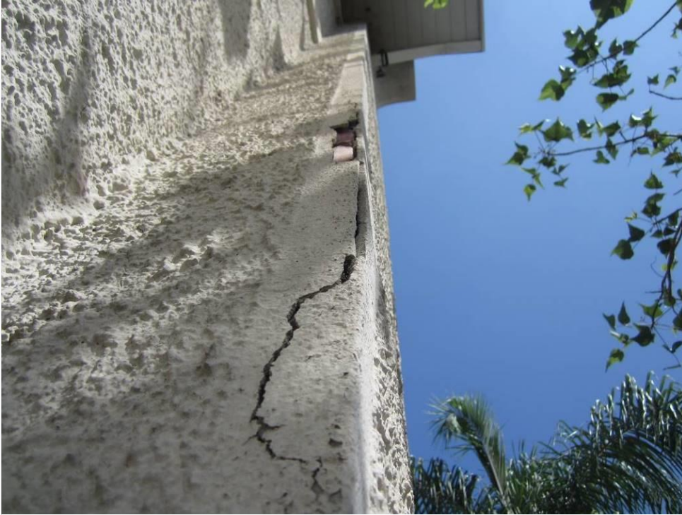
Photo 7 – Vertical crack leading to exposed brick masonry.
