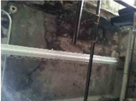
E-13: Fluorescent strip light wire guard in utility room
