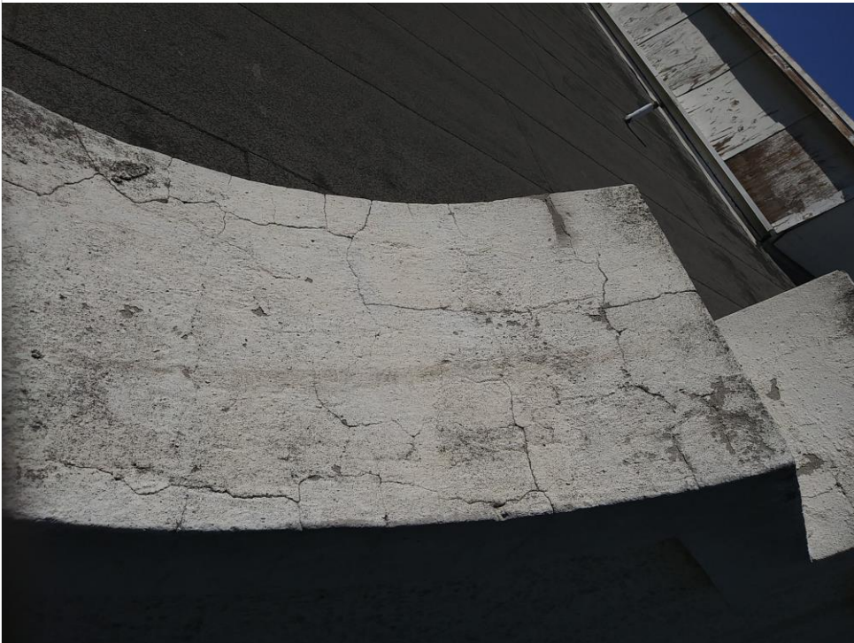
Photo 22 – Cracks at top of parapet wall.
