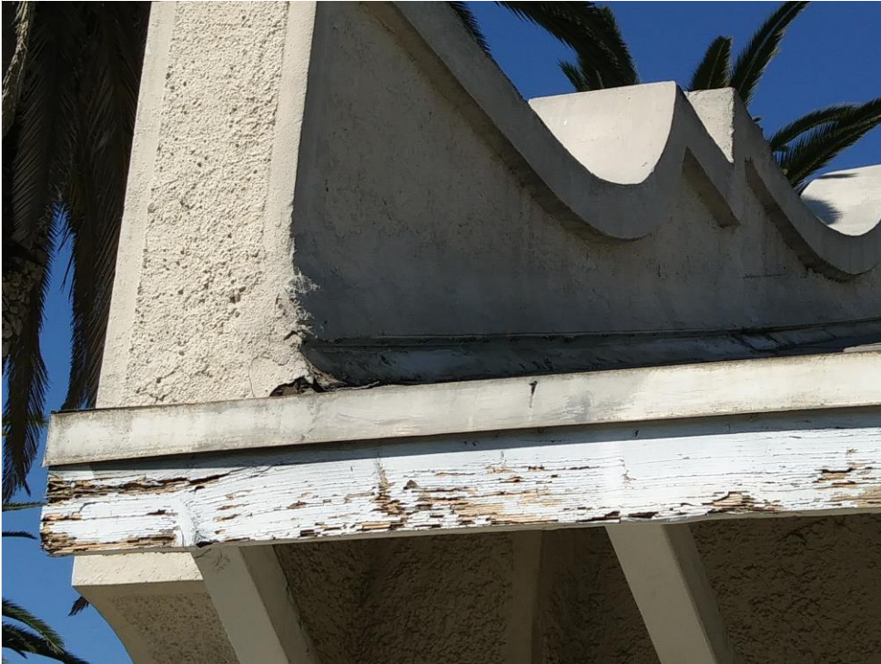
Photo 23 – Deteriorated wood fascia board at roof eave.
