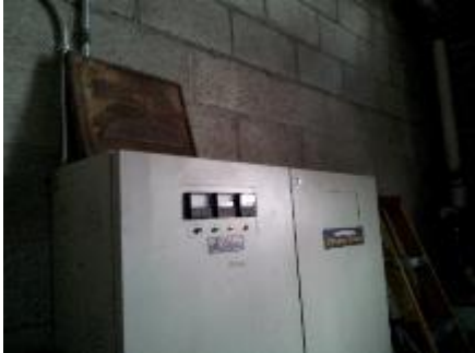
E-11: Inverter in use
