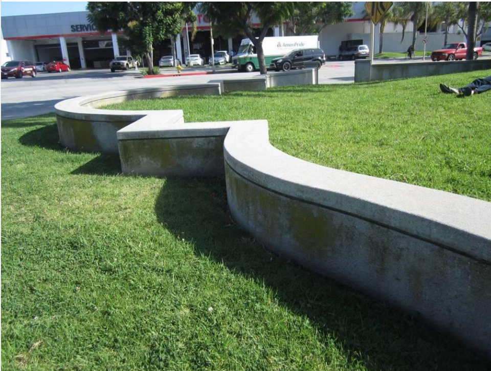
Photo 30 – Existing concrete landscaping walls with staining.
