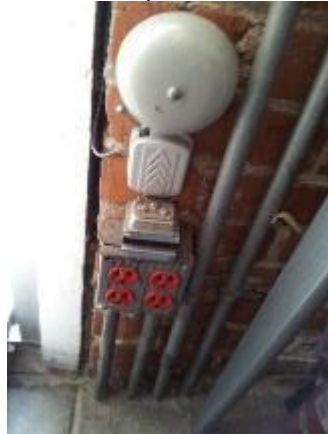
E-6: Fire alarm sprinkler bell and receptacle outlet
