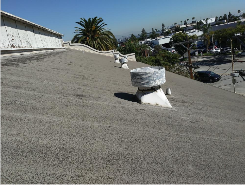
Photo 21 – Existing roofing membrane and vent penetrations.
