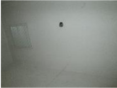
P-3: Existing recessed sprinkler head with no escutcheon
