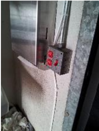
E-20: Outlet in 2 nd floor restroom
