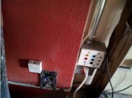
E-22: Open junction box in 2 nd floor office
