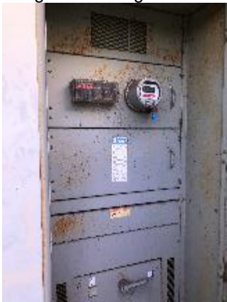
E-33: Main Switchboard
