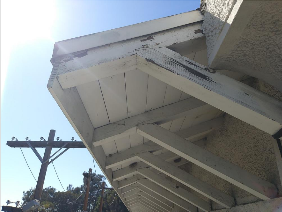
Photo 25 – Paint coating is worn at the edge rafters and diagonal struts that support the roof eave.
