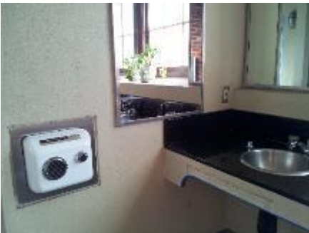
E-8: Hand dryer and GFCI in men's restroom
