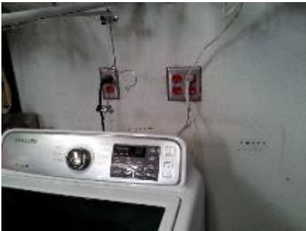
E-17: Outlets in use
