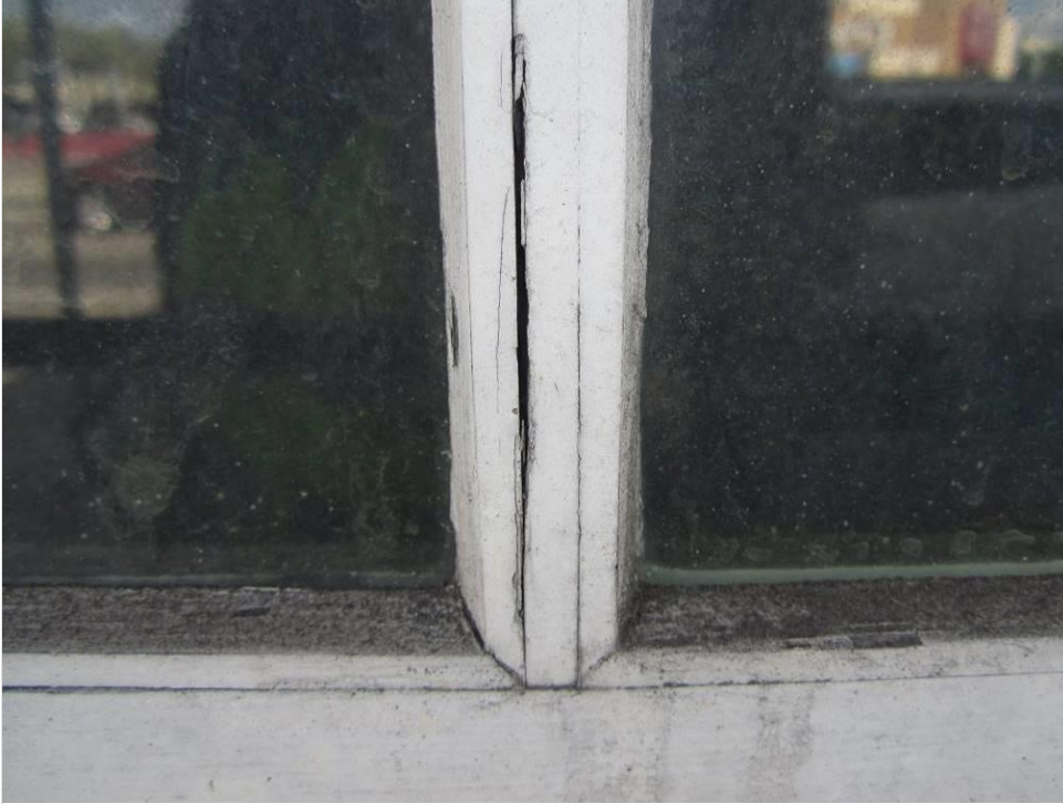
Photo 15 – Wood window muntin needs repair.
