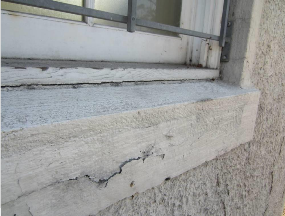
Photo 16 – Wood window sill and concrete ledger with crack in paint coating. Note that the joint between the wood sill and ledger is not sealed.
