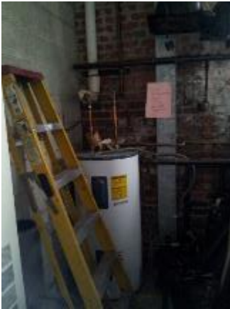
E-15: Electric water heater
