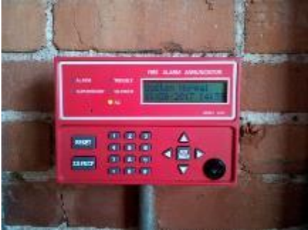
E-5: Fire alarm annunciator near front entrance
