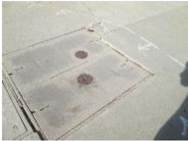
P-4: Structural damage to vault
