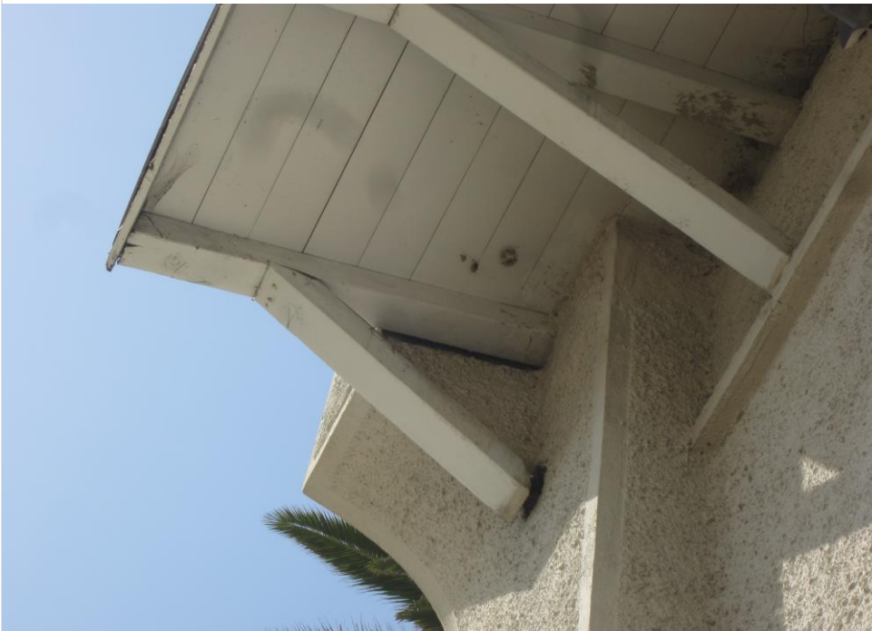
Photo 26 – Diagonal wood strut needs to be reattached to the wall. Gap between the wall and roof interface needs to be sealed.
