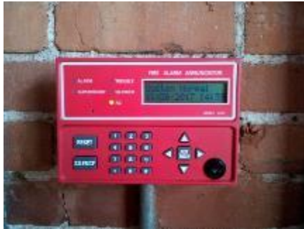
E-5: Fire alarm annunciator near front entrance
