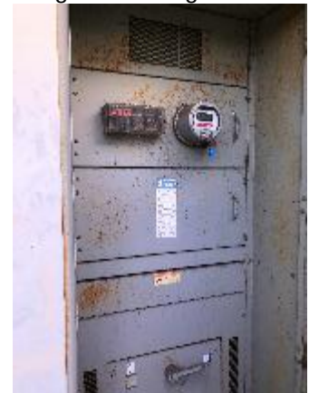
E-33: Main Switchboard
