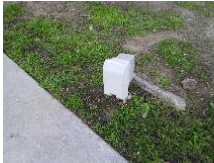
E-30: GFCI outlet near entrance not working
