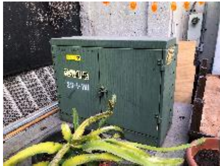
E-32: Utility Transformer
