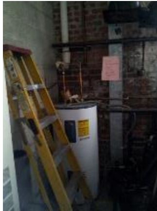
E-15: Electric water heater
