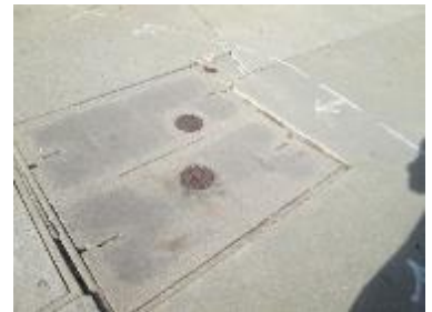
P-4: Structural damage to vault
