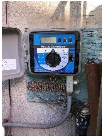
E-36: Exterior irrigation controller
