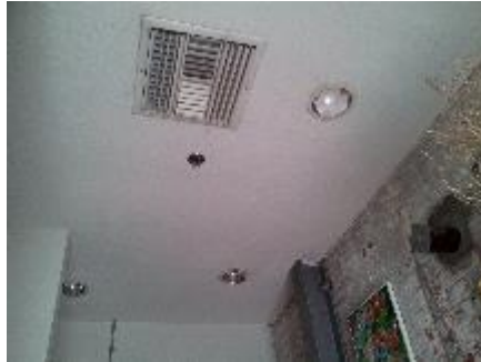
E-19: Downlights in 2 nd floor restroom
