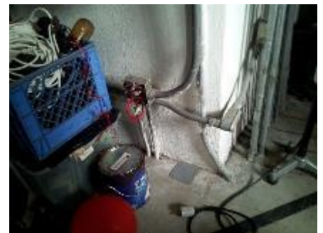
E-14: Open junction box in utility room
