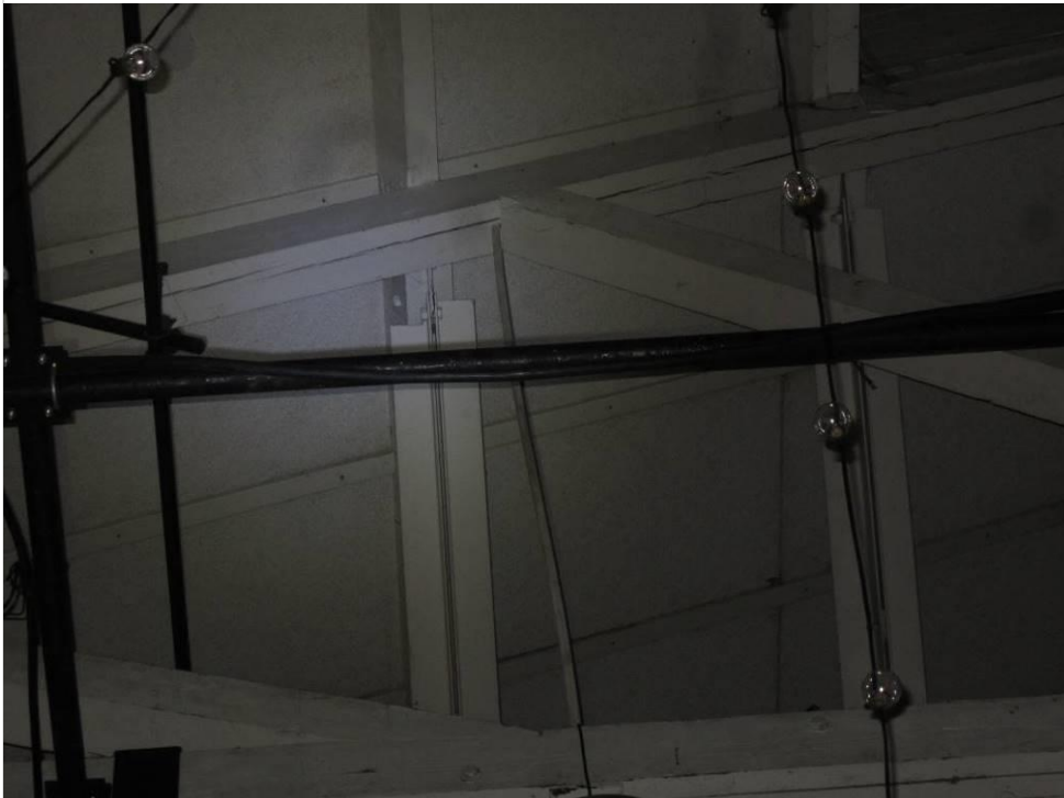
Photo 28 – Split in wood truss member.
