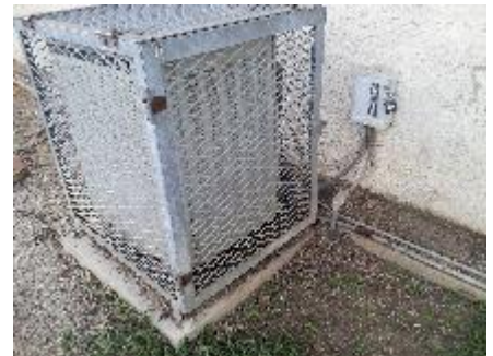
E-35: Exterior AC Unit with disconnect
