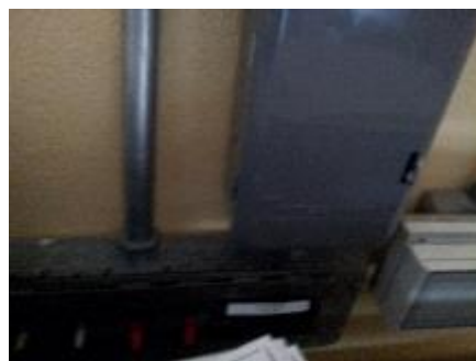
E-23: Switches in office room
