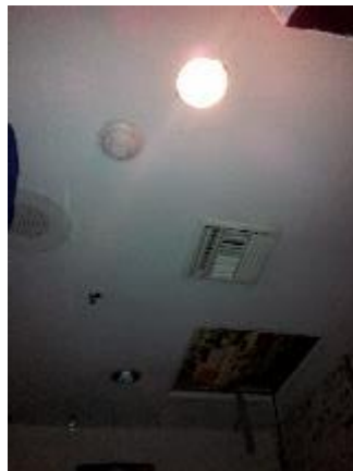
E-25: Recessed downlight in “dungeon” room
