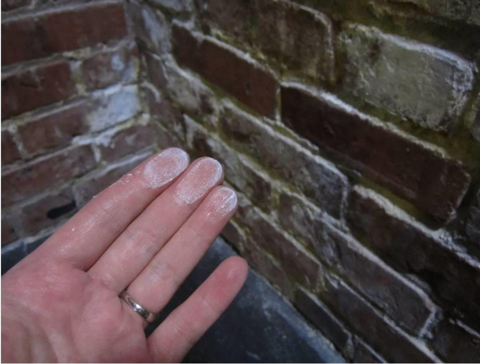
Photo 11 – Efflorescence at interior brick masonry wall.
