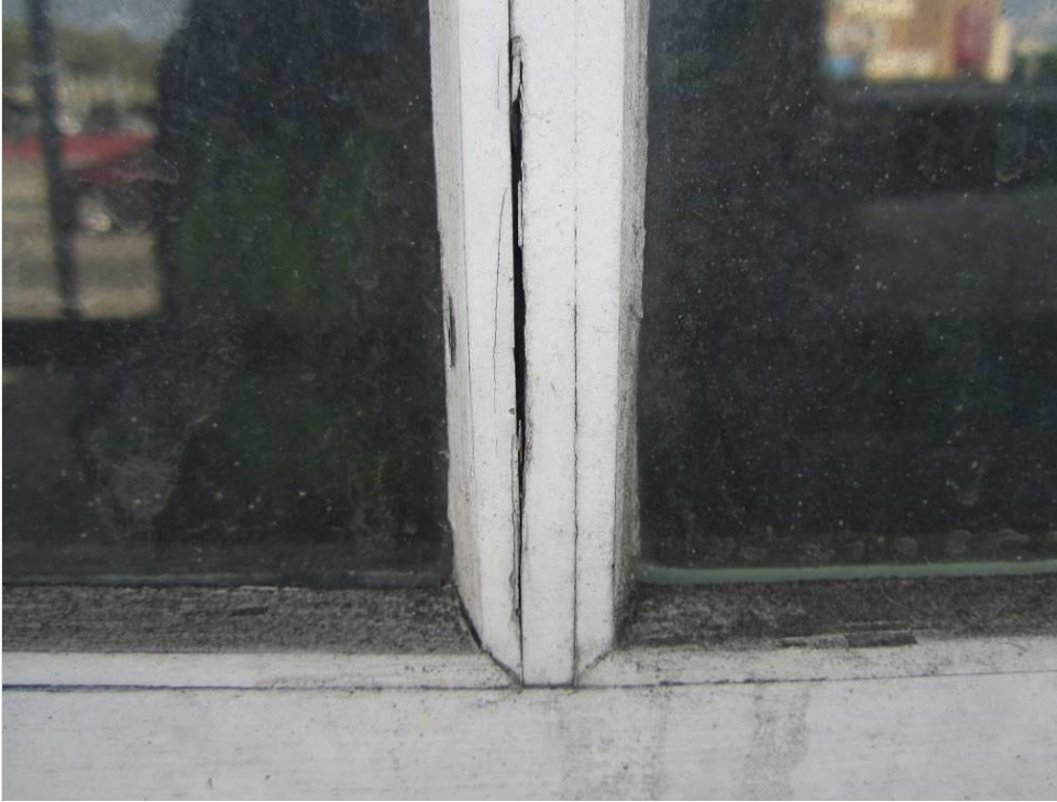
Photo 15 – Wood window muntin needs repair.
