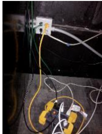
E-26: Quad outlet in control room
