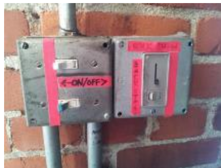
E-1: Light switches near front entrance
