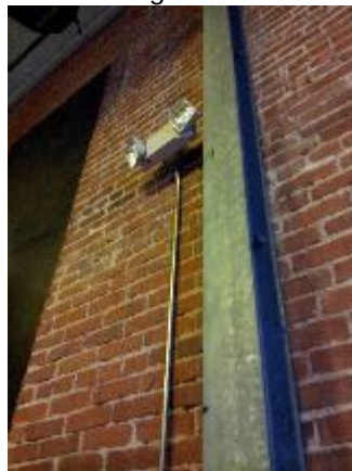
E - 29: Emergency lighting in performance hall
