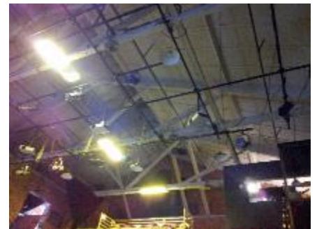
E-28: (3) 2x4 fixtures above seating area
