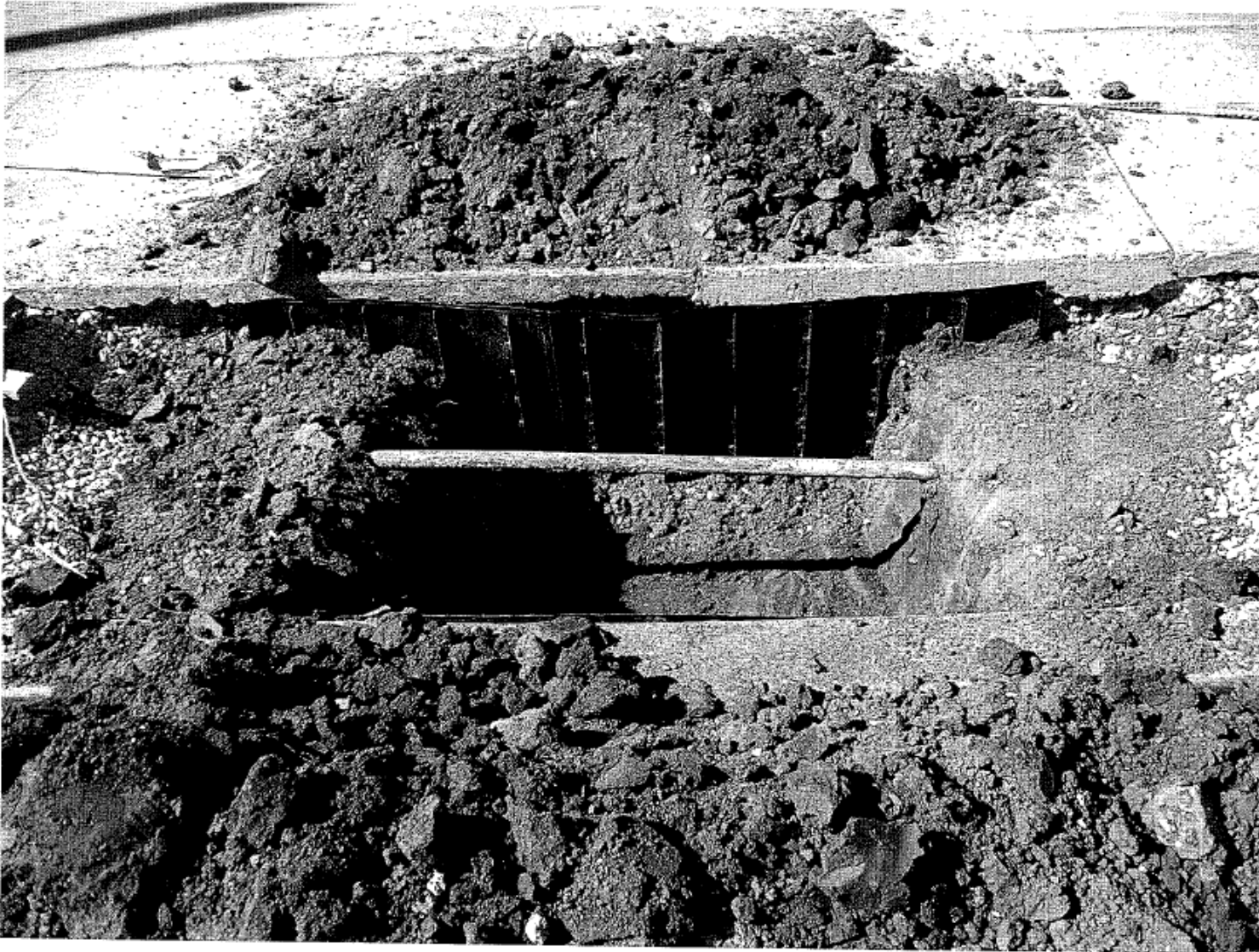
Above: Utility line runs directly through the middle of the proposed tree well, which prevents tree planting.
