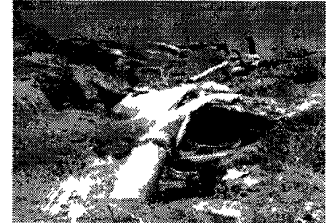
Bishop Montgomery Slope Failure City of Torrance California
