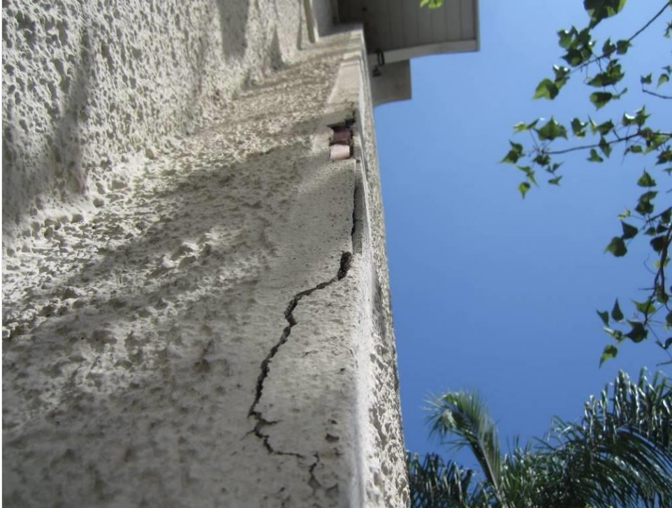
Photo 7 – Vertical crack leading to exposed brick masonry.
