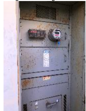
E-33: Main Switchboard
