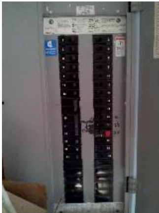
E-21: Panelboard "A" in office room
