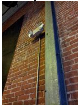
E – 29: Emergency lighting in performance hall
