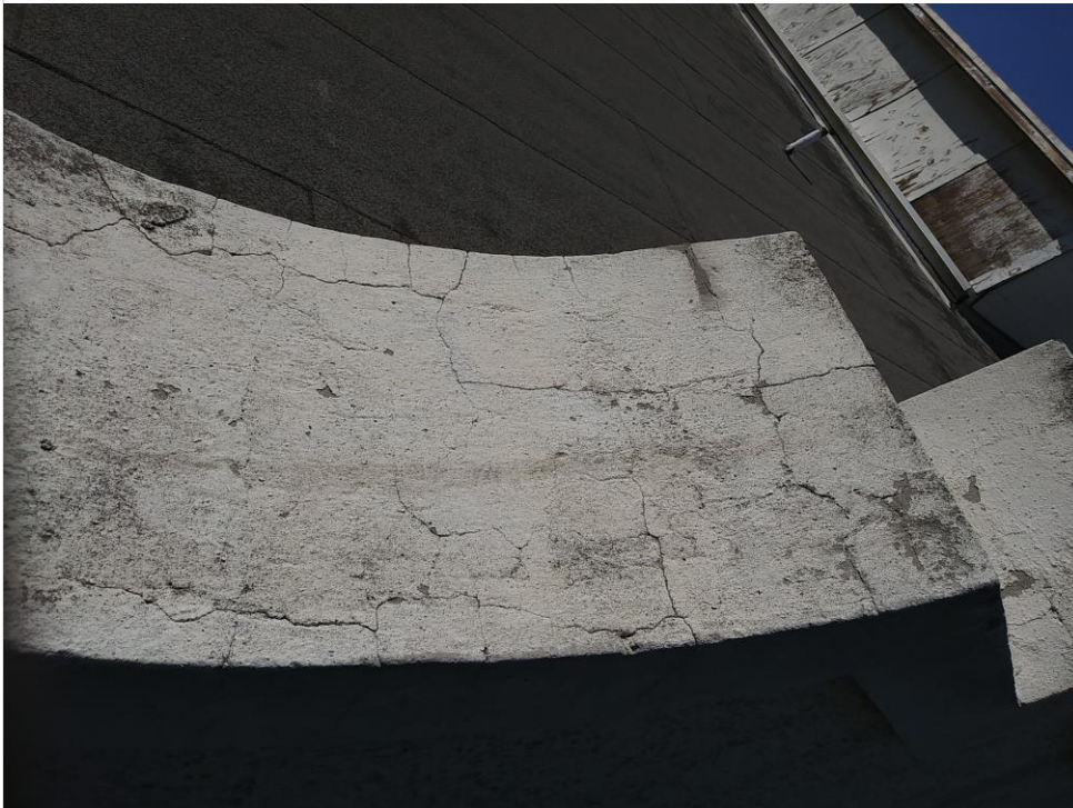
Photo 22 – Cracks at top of parapet wall.
