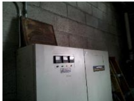
E-11: Inverter in use
