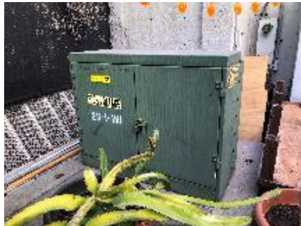
E-32: Utility Transformer
