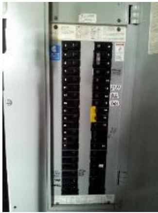
E-9: Panelboard "B" in utility room
