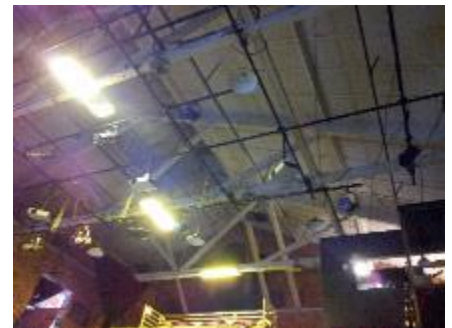
E-28: (3) 2x4 fixtures above seating area
