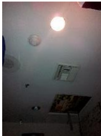
E-25: Recessed downlight in “dungeon” room
