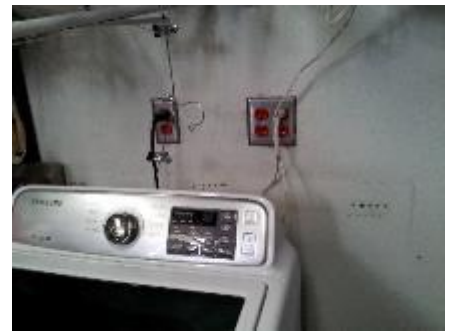
E-17: Outlets in use
