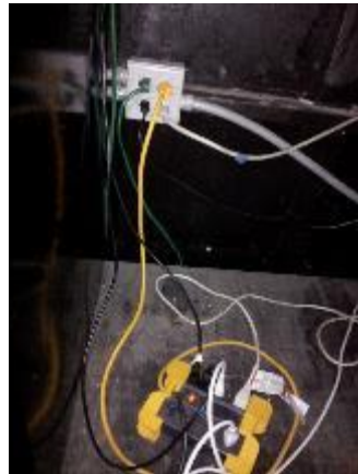
E-26: Quad outlet in control room
