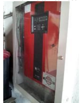
E-12: Fire Alarm Control Panel
