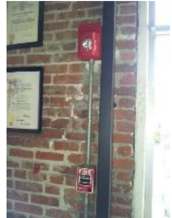
E-4: Fire alarm pull station and strobe
