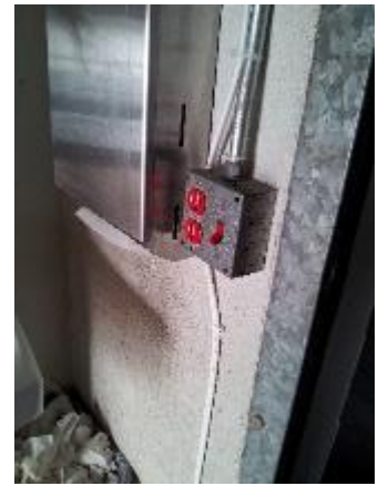
E-20: Outlet in 2 nd floor restroom
