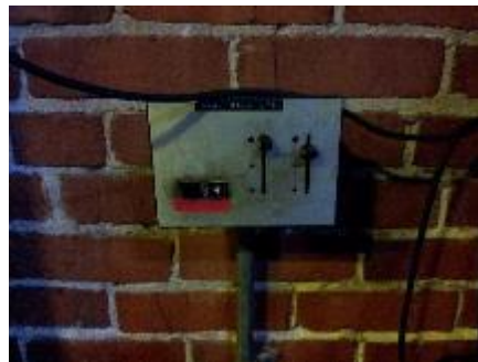
E-27: Dimmer switch controlling (5) 2x4 light fixtures
