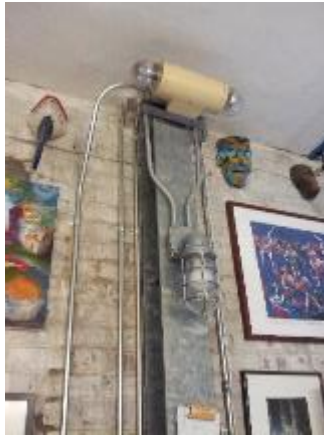
E-24: Emergency lights in open office area
