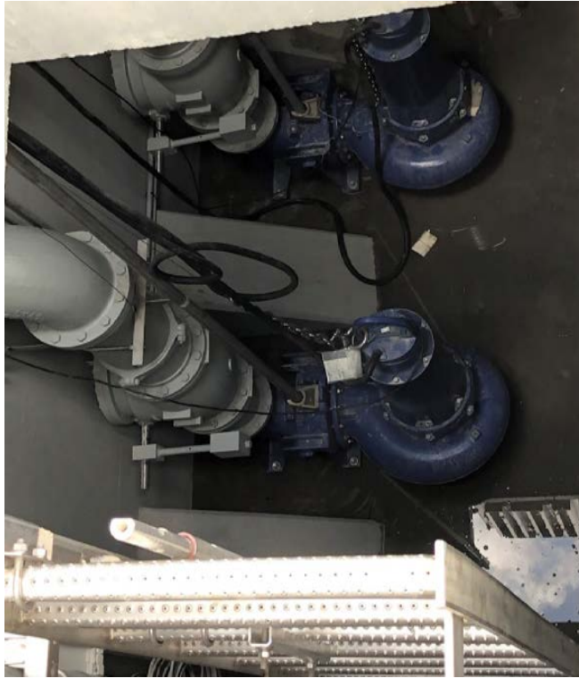
Figure 3-5. Example Stormwater Pumps Installed in a Wet Well
