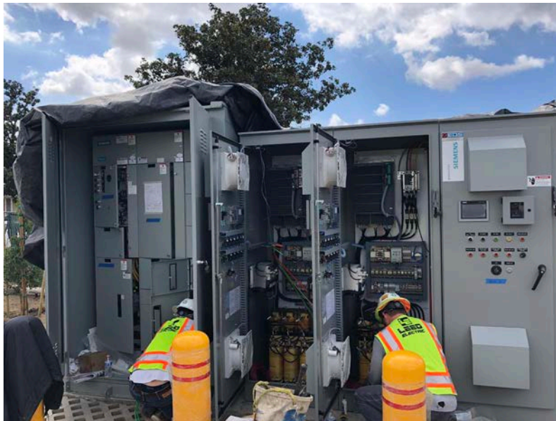
Figure 3-6. Example Pump Station Control Panel
