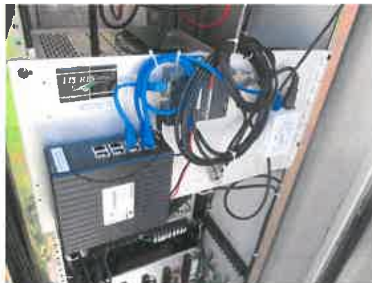
Figure 11 – AP Equipment Panel in Type 332 Traffic Cabinet
