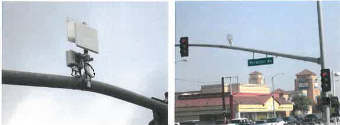
Figure 10 – Typical WLAN Access Point Equipment Installations
