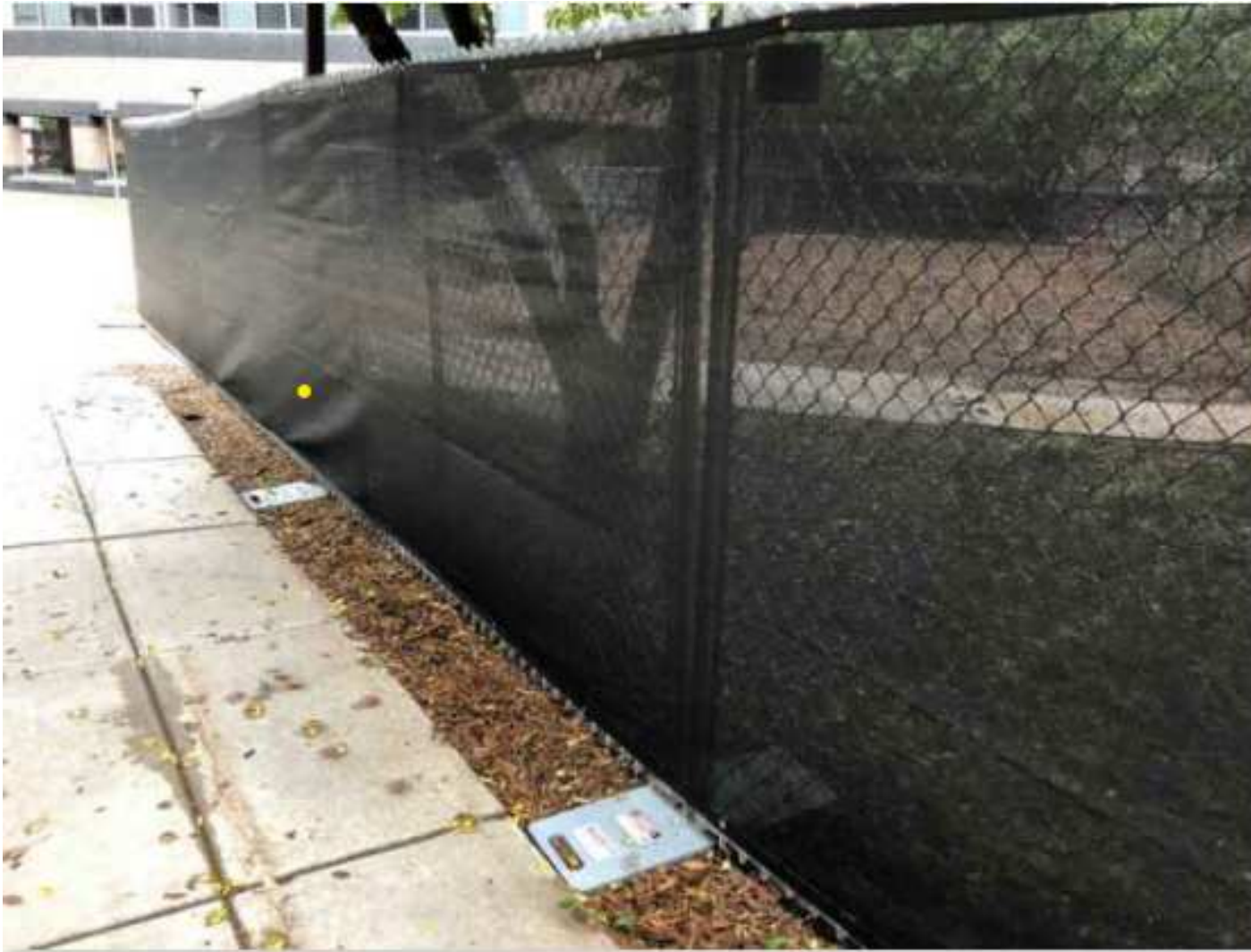
EXAMPLE OF CHAIN LINK SAFETY FENCE WITH PRIVACY SCREEN USED FOR PERIMETER CONTROL.
