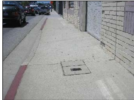
RECONSTRUCT DRIVEWAY TO MEET ADA REQUIREMENTS.
