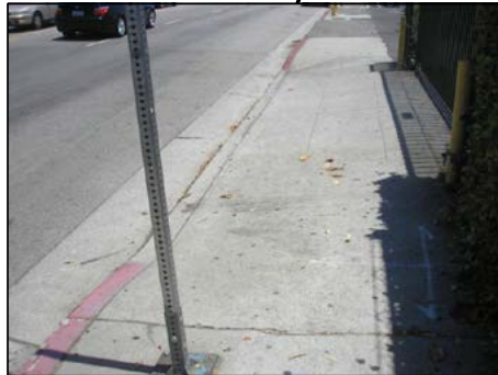
RECONSTRUCT DRIVEWAY TO MEET ADA REQUIREMENTS.
