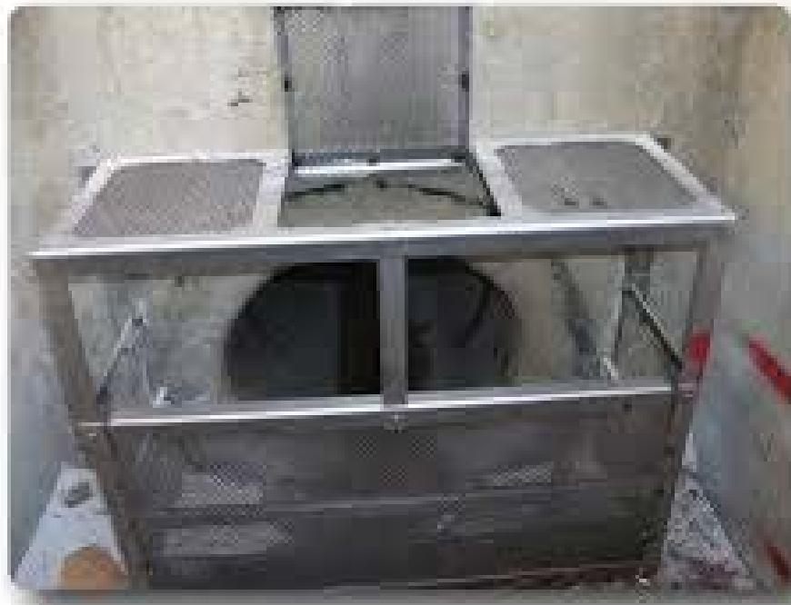
Connector Pipe Screen (CPS) Inside Catch Basin
