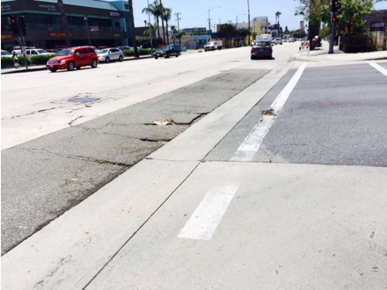
Figure 4. Valley gutter slopes and pavement conditions exiting Costco. Photo courtesy of Barry Kurtz.
