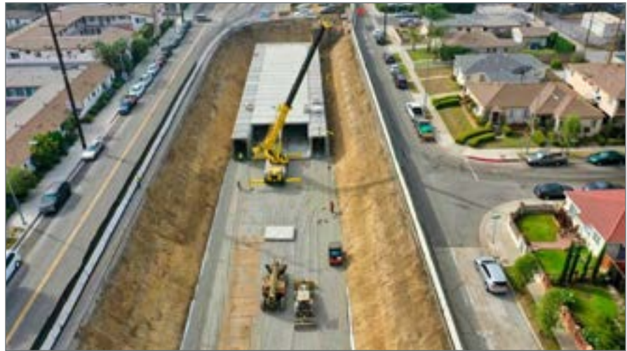
Culver Boulevard Realignment and Urban Runoff and Stormwater Project. Source: Michael Baker Intl.
